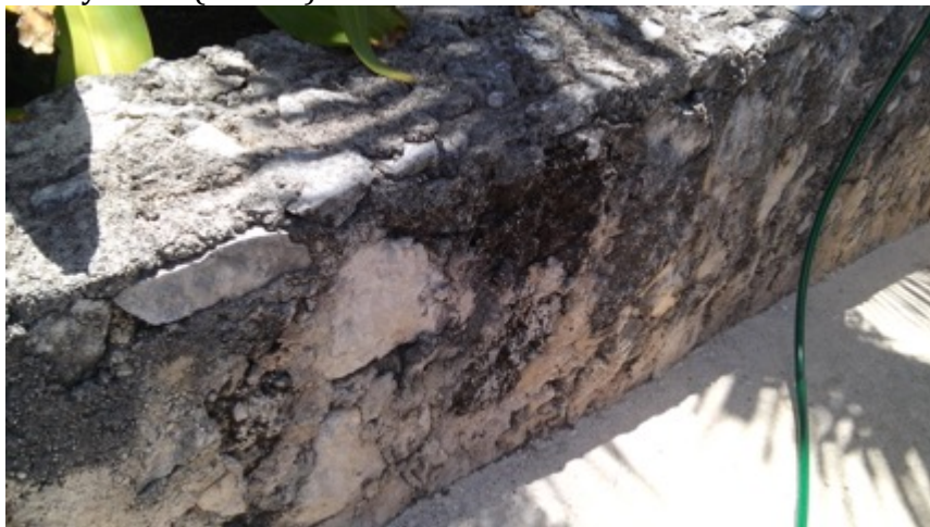
Moldy walls (Before):
