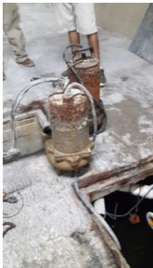
- Second and larger Sump Pump for north garage failed. Replacement has been ordered -
