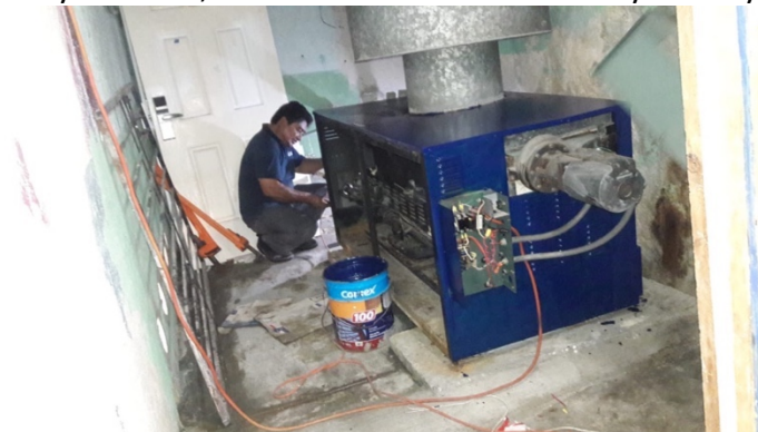
Pool heater 100% ready.
