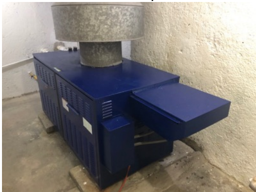
Added a Motion Sensor Light to illuminate the area by Elevator #4: It was very dark on some afternoons and cloudy days.
