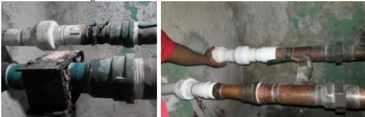
-Pool Heater Plumbing-
