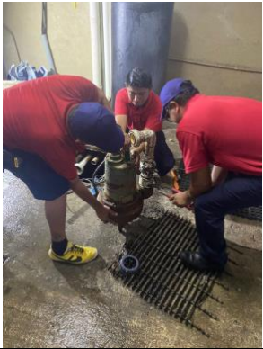
General Plumbing Preventative Maintenance:
