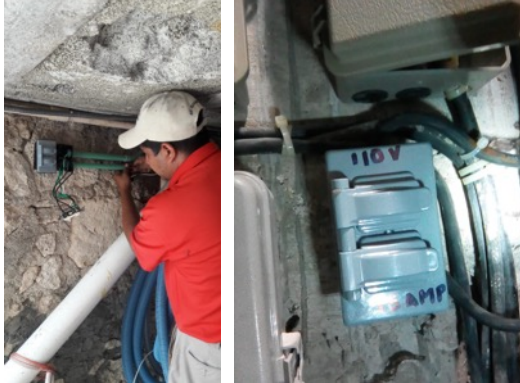
Installed Astronomic Timers:
