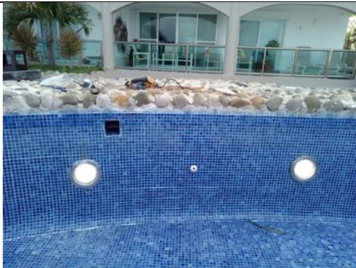
Repaired Camera Systems:
